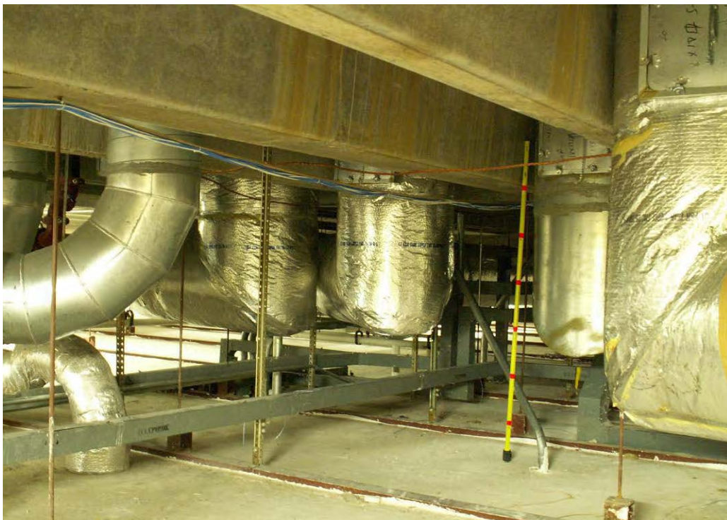
Photo B-6 Interior Service Module Showing ducts to interstitial service zone from penthouse
