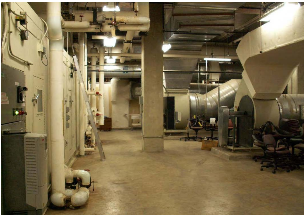
Photo B-4 Typical Service Bay
