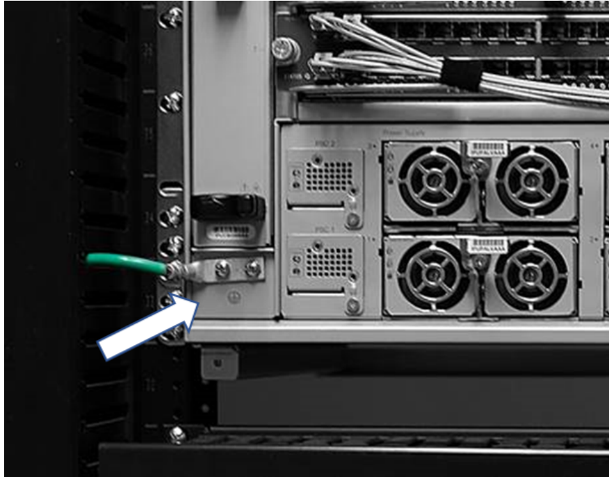
Figure 16: OEM Equipment Ground Connection
