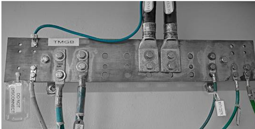
Figure 17: Primary Bonding Busbar
