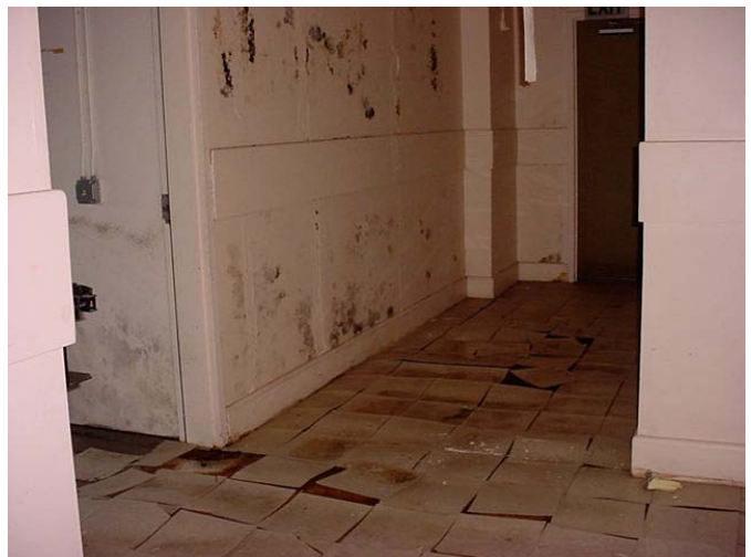
Photo 12 – water damage – level 2 – s. hallway
