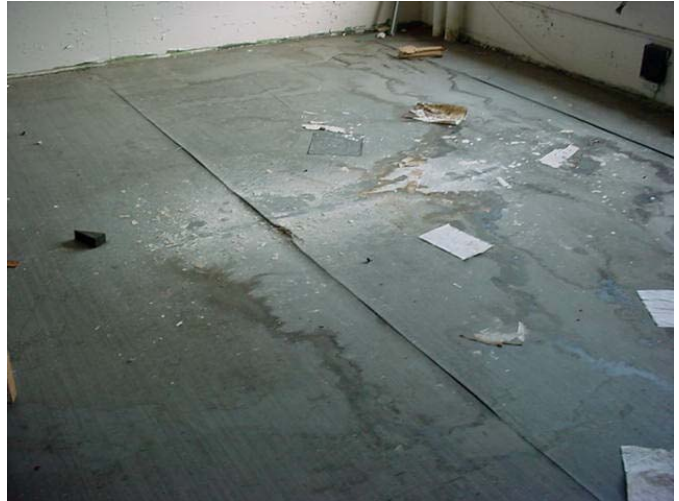
Photo 16 – water damage – level 2 – SEC room
