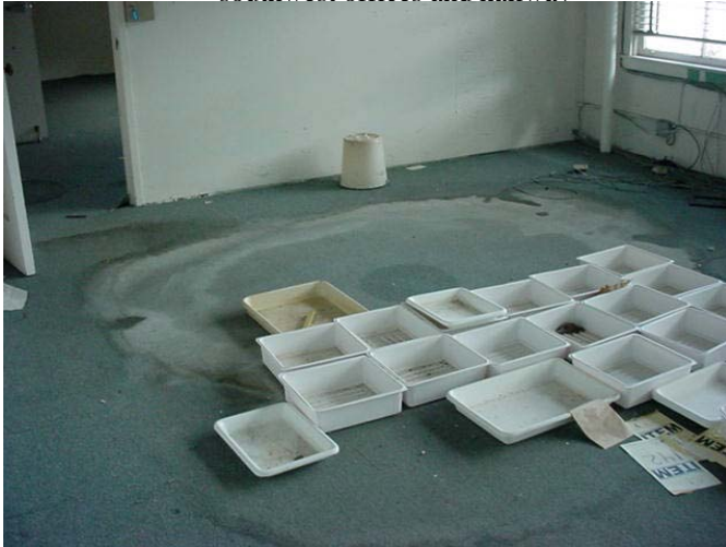
Photo 15 – water damage – level 2 – room 220
