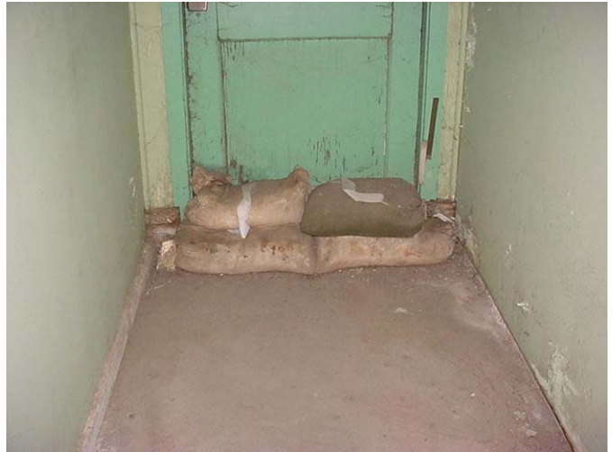
Photo 4 – water damage – level 1 – wood doorway
