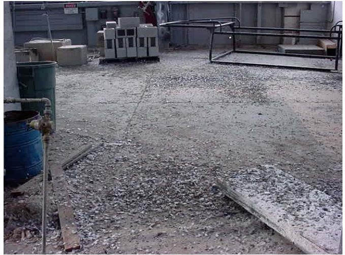
Photo 2 – bird droppings – level 1 – north side
