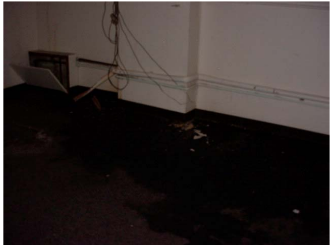
Photo 10 – water damage – level 2 – carpet – south side
