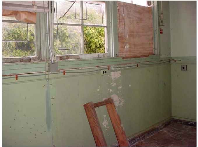
Photo 8 – level 1 – broken windows – water intrusion
