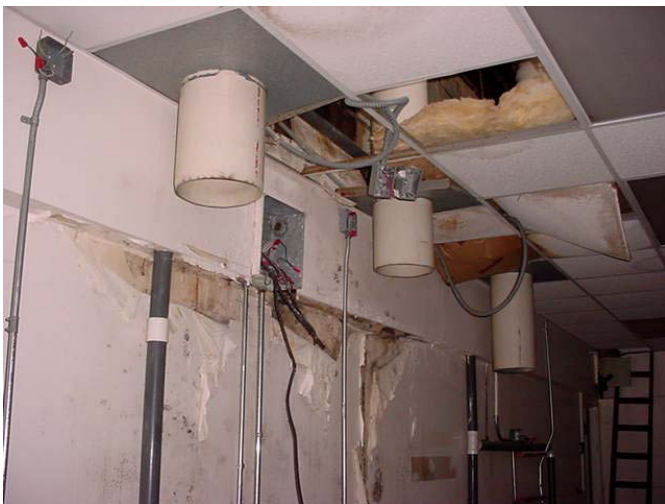
Photo 11 – water damage – L2 – Chemical Analysis Rm.
