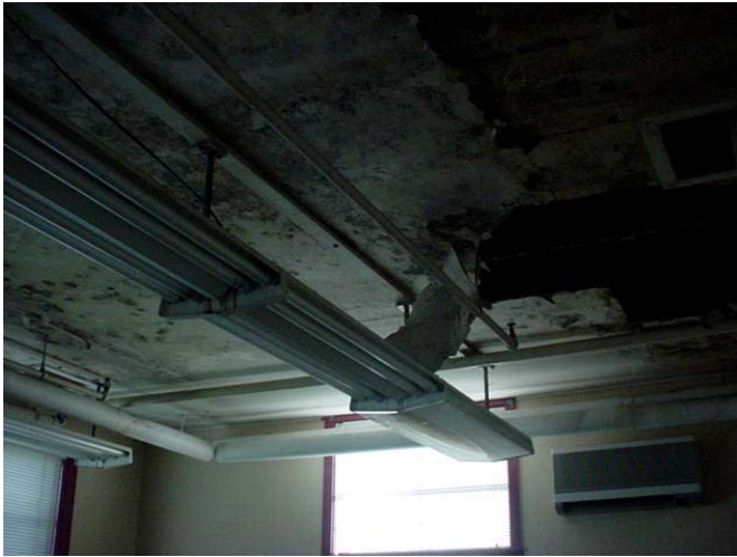
Photo 7 – water damage & significant growth – level 1 – engineer’s office
