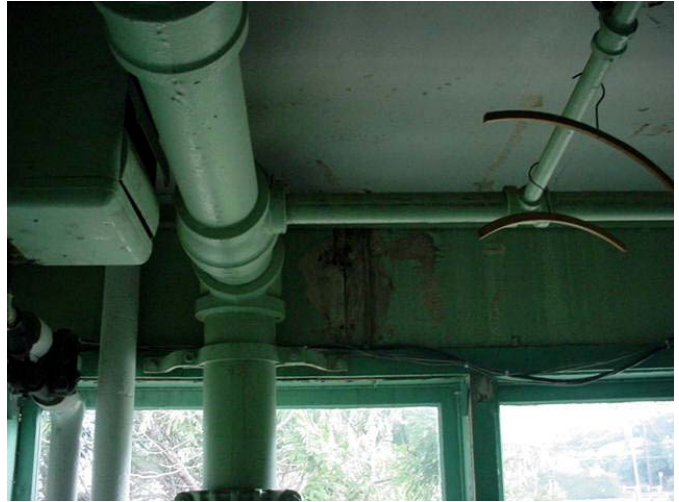
Photo 14 – water damage – level 2 – copy room
