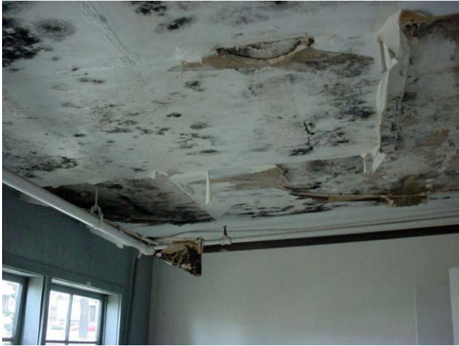
Photo 13 – water damage & significant growth – level 2 – southwest offices and hallway
