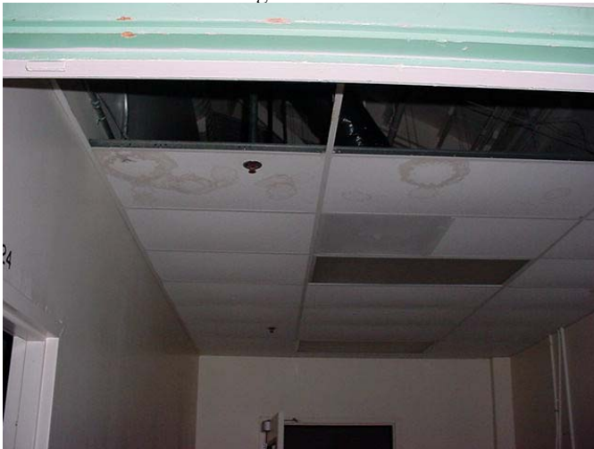
Photo 9 – water damage – level 2 – west ceiling tile
