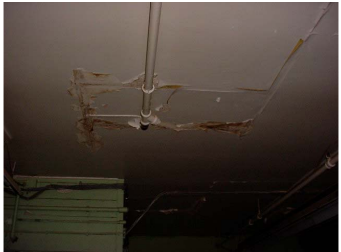
Photo 6 – water damage – level 1 – south sheet rock ceiling
