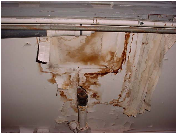
Photo 5 – water damage – level 1 – SE sheet rock ceiling
